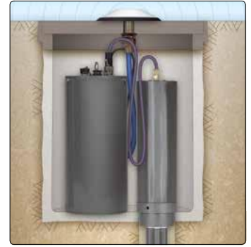
• Model 8026 Datalogger and Model 1150 (A-3) Extensometer in manhole.
