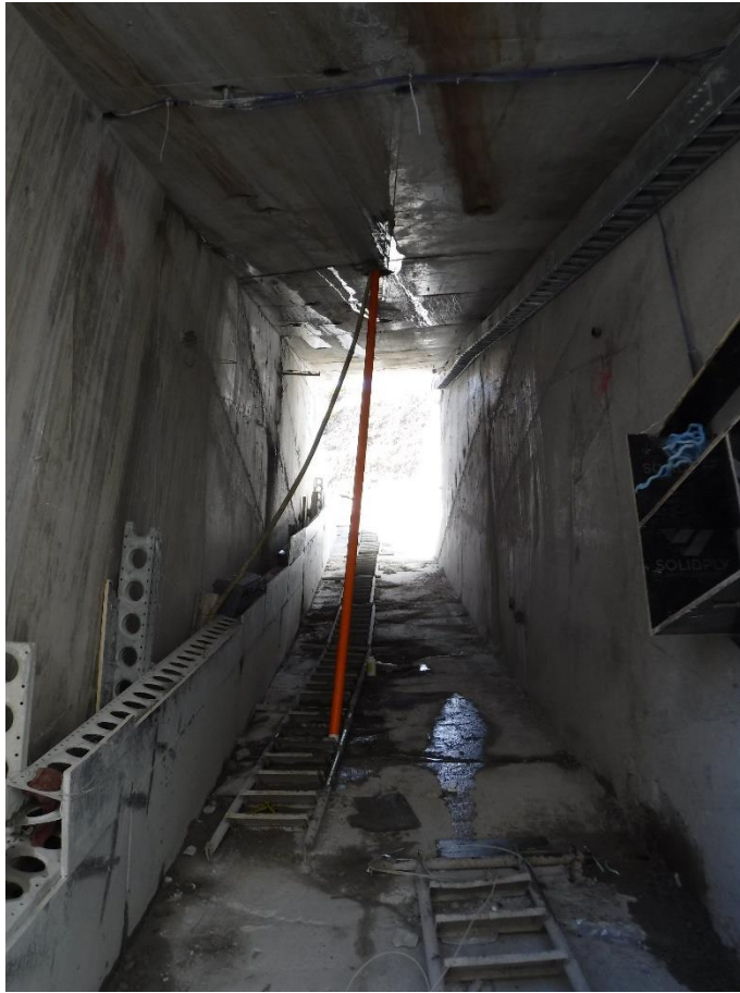
Figure 2 View from inside the gallery where inclinometer casing is being installed. The casing is slid through the roof of the gallery after which a worker will go and insert in the borehole in the floor of the gallery.
