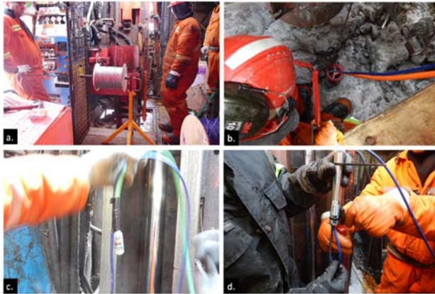
Figure 7. Instrumentation in Deep Boreholes: a. Air craft cable spool, b. Instrumentation cables at collar with securing tool, c. Thermistor String Sensor, d. Vibrating Wire Piezometer
