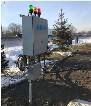
Visual warning system
