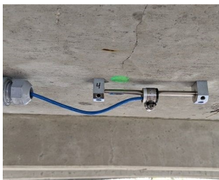
Vibrating wire strain gauge attached to the bottom flange of a girder
