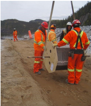
Upstream Horizontal SAAS Installation.
