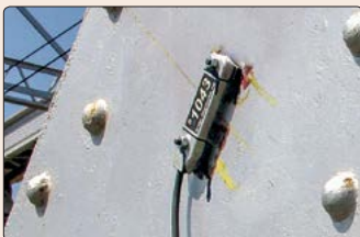
• Model ST-350 attached to steel truss.
