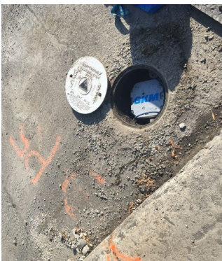
Extensometer data logger, hidden in a service box
