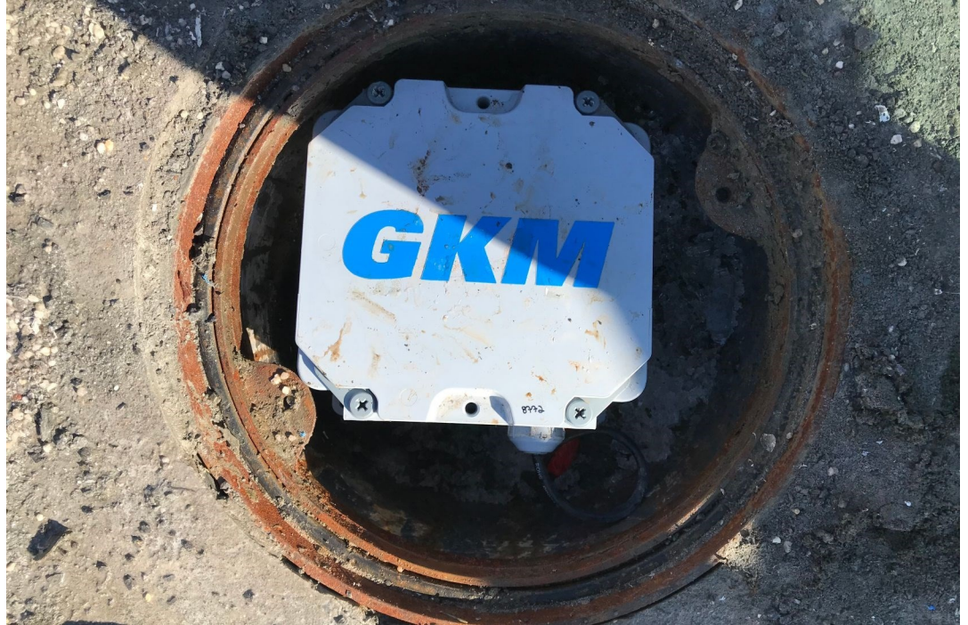
Real-time data acquisition system, integrated in a service box
