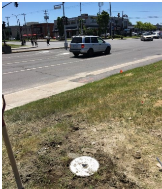
Surface monitoring instruments hidden in service boxes
