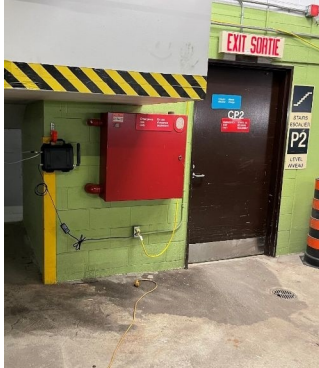
INFRA D10 connected to multiple sensors, to monitor sound and noise
