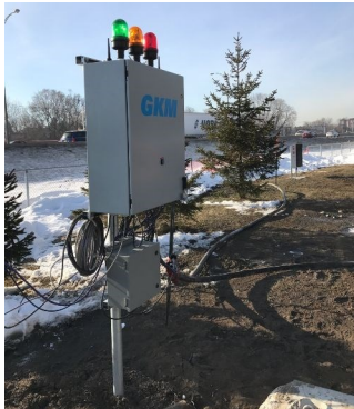
Visual warning system
