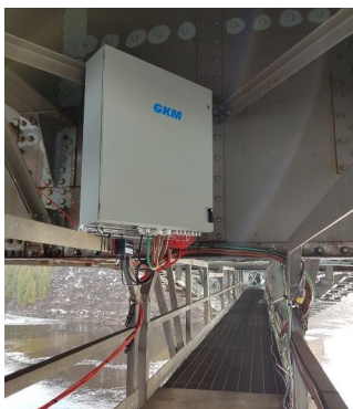
One of the two custom-made data acquisition systems installed under the Alexandra bridge.
