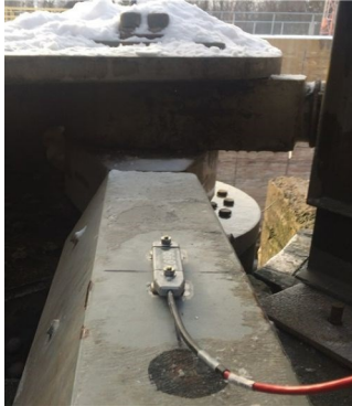
Strain gauges on the gates mechanisms to track dynamic strain during operations
