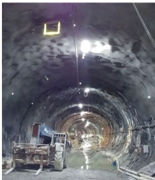
Instrumented shotcrete tunnel liner section
