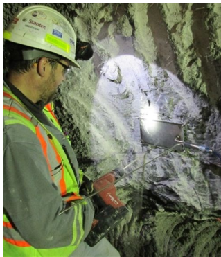
NATM pressure cells installed at the interface of the shotcrete tunnel liner and natural ground
