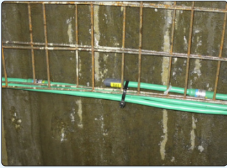
• Temperature measurement profile with thermistor strings installed along circumference of the frozen soil
