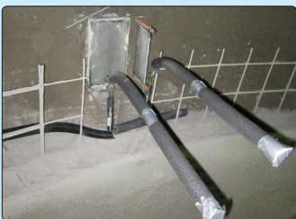
• Geokon 4850 NATM radial and tangential pressure cells installed at the interface of the ground and shotcrete lining
