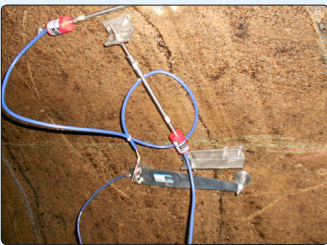
• Typical 3D crackmeters and geophone installation in tunnel
